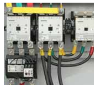
Wye-Delta reduced voltage starter uses all Siemens components.
